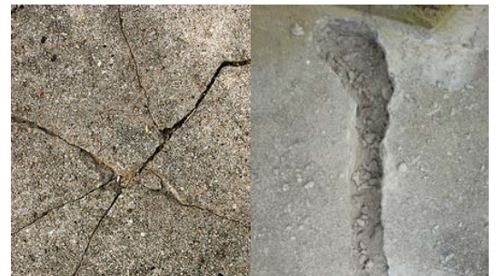
It might seem to be just a little crack from the surface, but it could be a big hole inside already!
