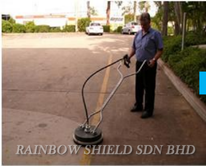
Apply Mouldshield C and clean the concrete surface with high pressure water jet
